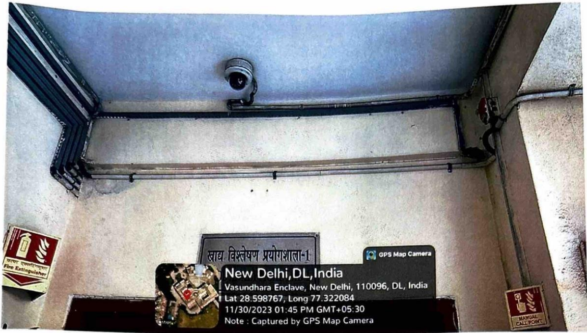
CCTV cameras ensure the security of the campus
