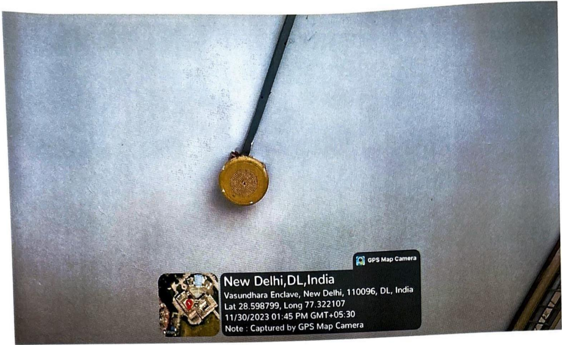
Fire alarm sprinkler system
