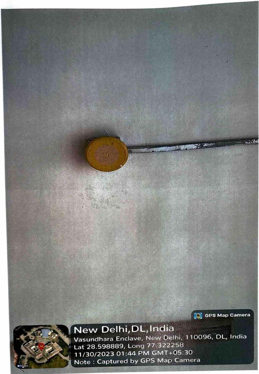
Fire alarm sprinkler system
