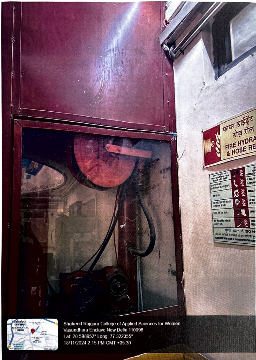
Fire hydrant and hose
