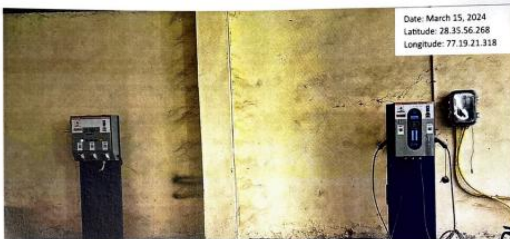
EV charging station
