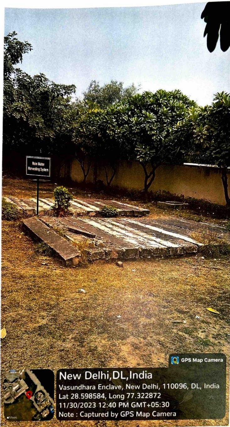
Rainwater harvesting pits
