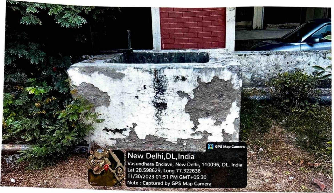
Water storage tanks
